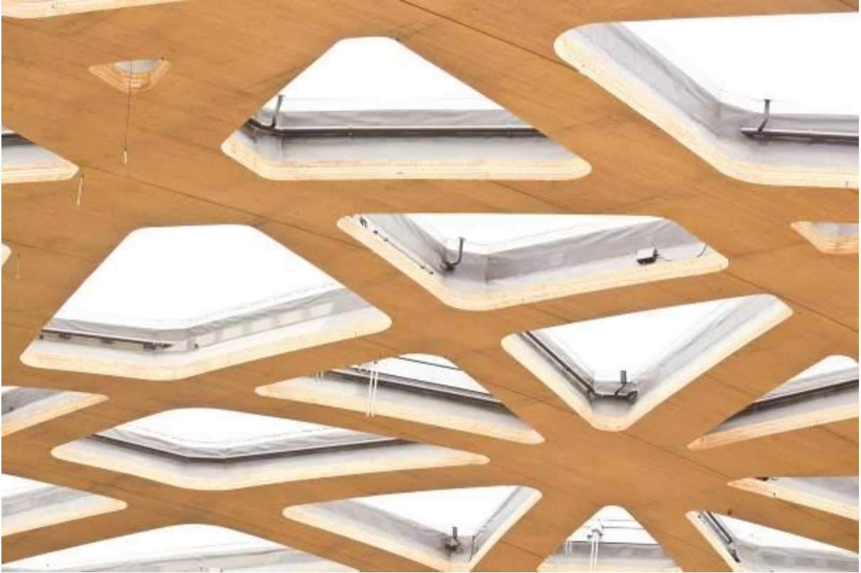
The roof structure allows plenty of light to filter into the interior of the elephant house.
